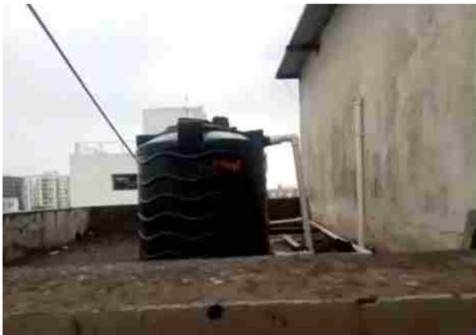
Water storage tank on roof
