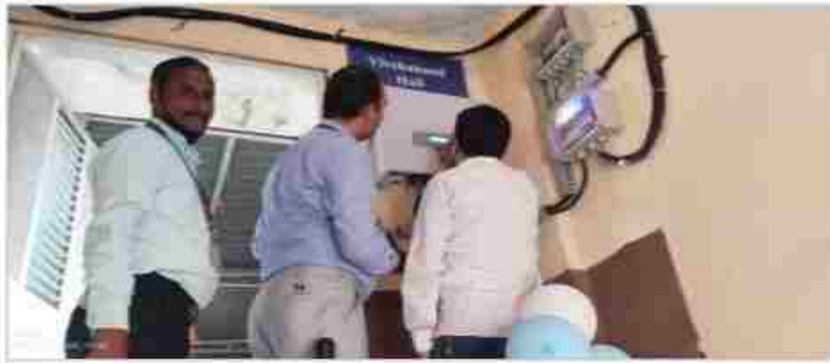
Net metering device in the premises
