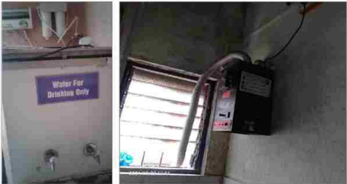
Sanitary vending and disposal machine is made available in premise including water facility
