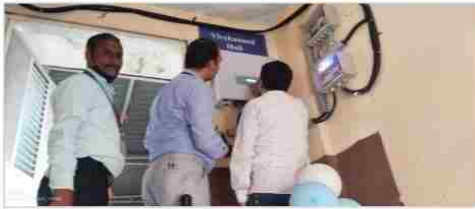
Net metering device in the premises
