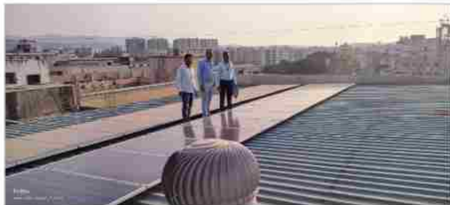
Energy efficient fan and solar roof top
