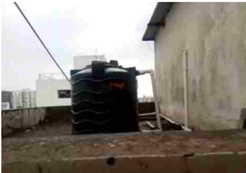
Water storage tank on roof
