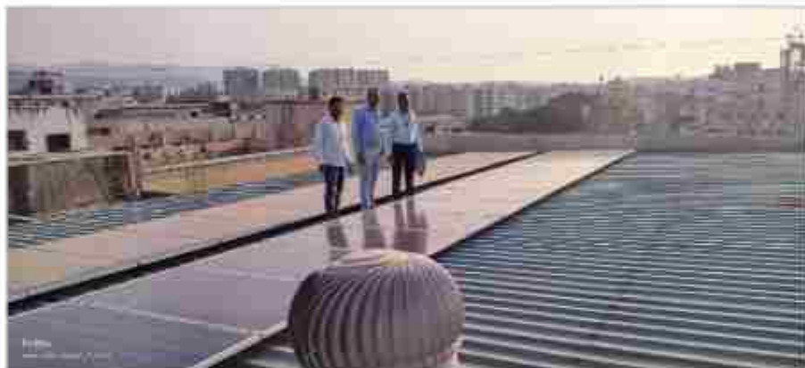
Energy efficient fan and solar roof top
