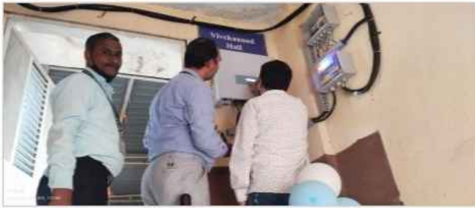
Net metering device in the premises
