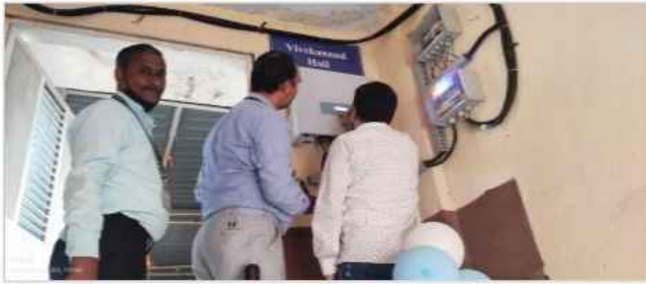
Net metering device in the premises
